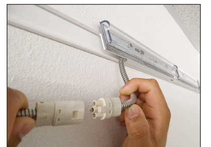
Figure 9 Connect the first fixture(s) to the power feed cables with the supplied tool-less connectors. Connect pr1meFX runs together using same tool-less connectors.
